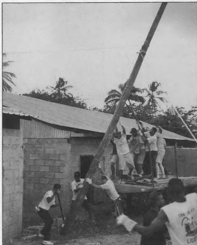
Workers set a pole the old-fashioned way, by hand. Kyle is standing just under the pole, helping guide it into the hole. The men set five poles in just 40 minutes.
