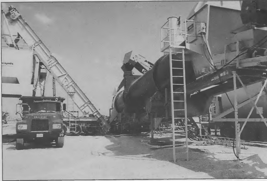
The plant is modern and state-of-the-art, and is highly portable; note the wheels on the conveyor unit in the background.
