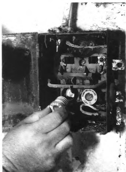
Fuses such as these are no longer in widespread use, having been replaced by breakers.
