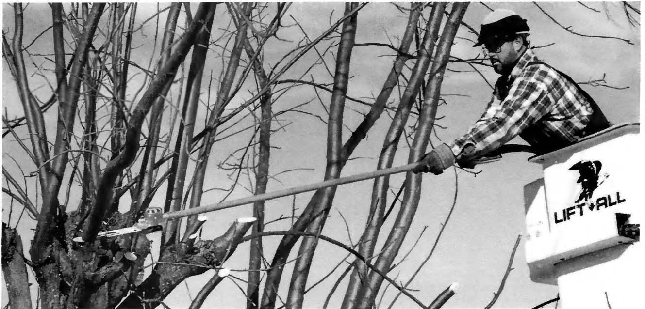
Gregg Cotten, line clearance foreman, uses a hydraulic saw to cut a limb out of lines.
