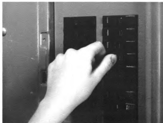
Breakers such as these are more convenient than fuses: if they trip often, you still have problems.
