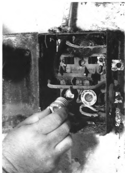
Fuses such as these are no longer in widespread use, having been replaced by breakers.
