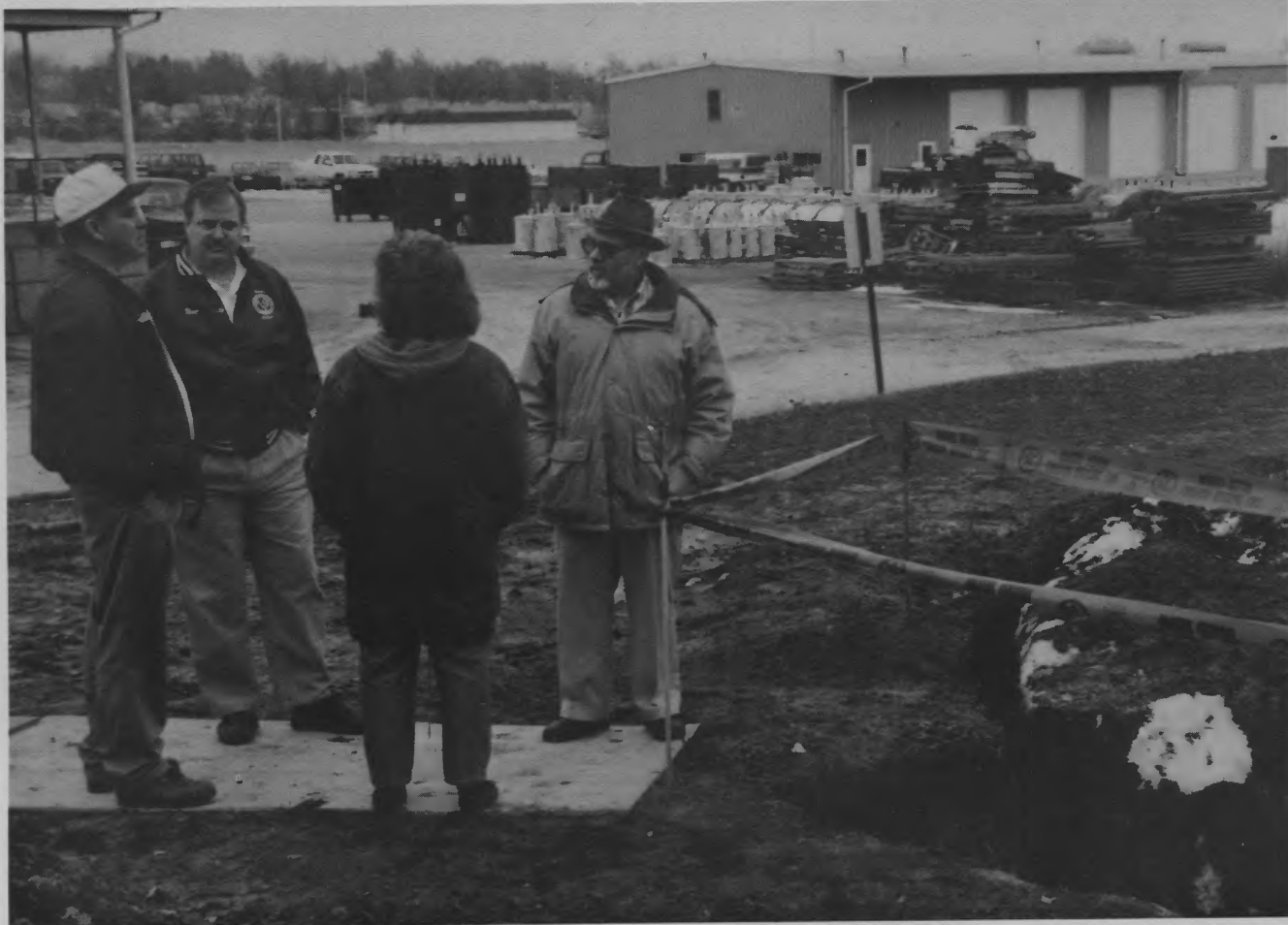
The heart of a geothermal system is a grid of buried pipes holding fluid that circulates through the system. Here, EIEC employees have a look at trench. From left are Tim Frick, Wm. David Champion, Jr., manager, Merrily Griffin and Dick Haines.
