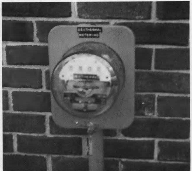
A typical meter for the geothermal system.
