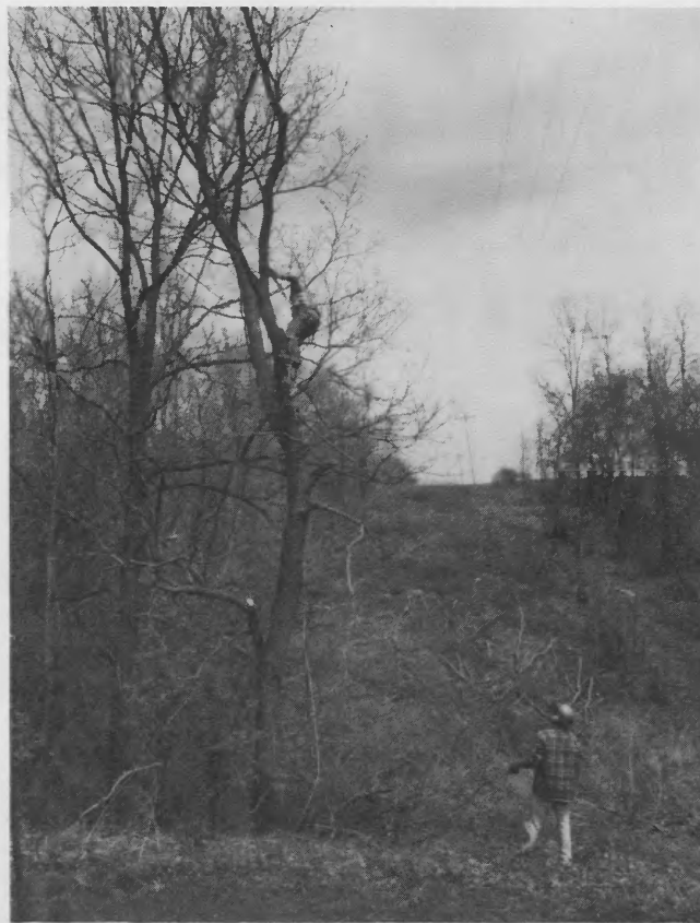
Chuck Cook and Tim Bussan of Stetters tree service cut down the tree that is in the power line right-of-way.
