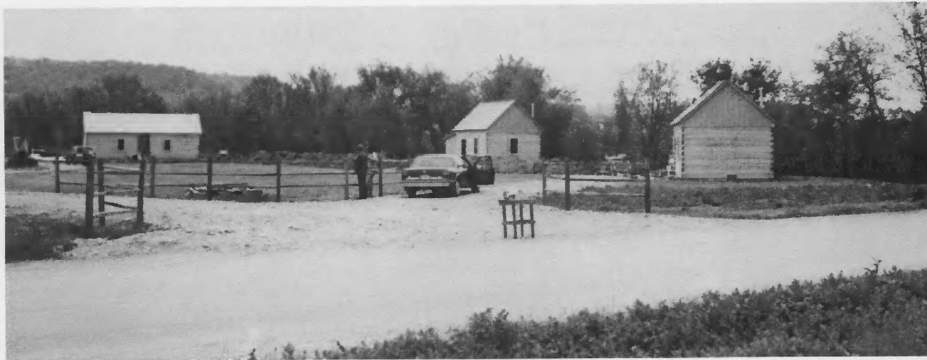
Four of the cabins are built, with the foundations in place for the other four cabins.
