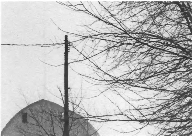
A future problem: These overhanging limbs will soon be in the service wires. Help us prevent a problem. Notify your Outside Operations office so we can schedule trimming when time permits.
