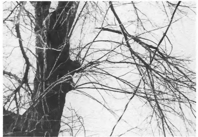
These wires are in danger from broken limbs resting on the line. Trimming could have prevented this power loss.
