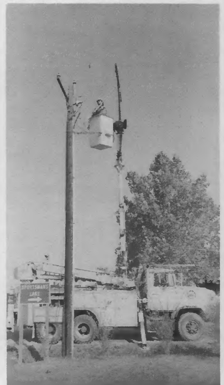
Lineman Gary Albers, high in the sky, disconnects a tap and raises a three-phase line to allow Moorehead's home to pass under.
