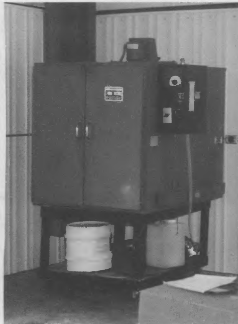
The oven in the recloser building which is used to dissipate moisture and solvents after equipment has been conditioned.
