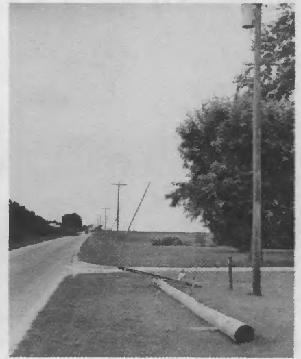
A new pole is ready to be put into service. The old line is "leaned" in the background.
