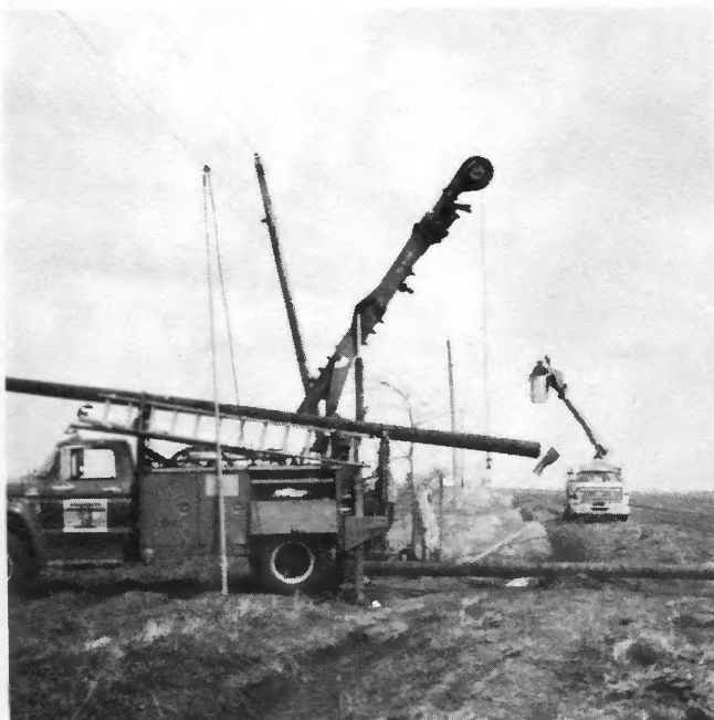
When replacing the conductor wire all poles are inspected. The bad poles are replaced.
