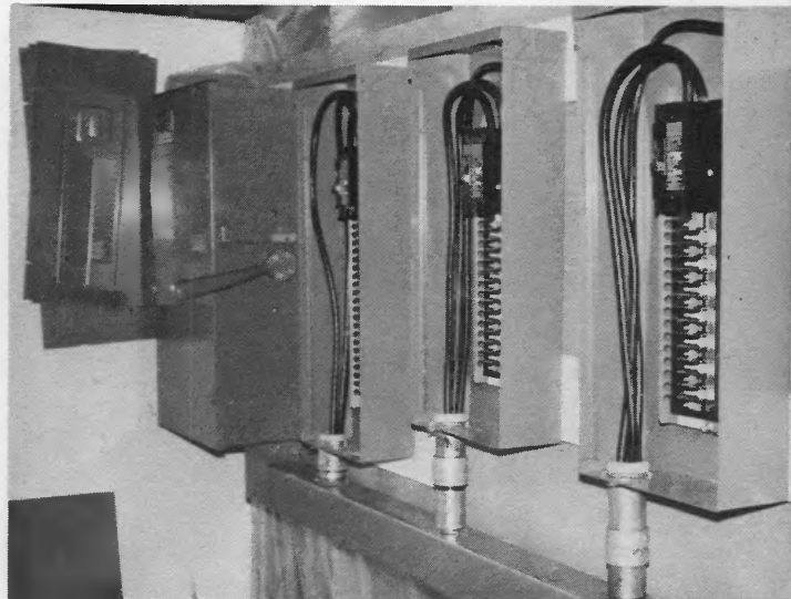
When standard metal service equipment is used, locate it in a clean dry room adjacent to livestock rearing area. Conduit should enter side or bottom with ends sealed.
