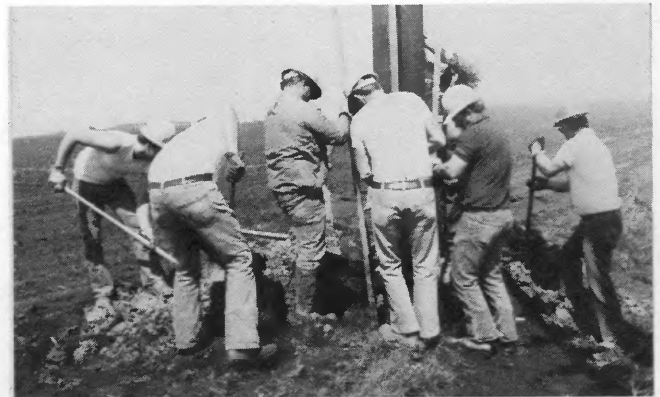
Crewmen tamp the earth around the new pole to make sure it is set securely.
