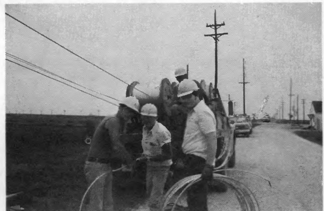
After the poles are securely in place, crews begin the task of stringing wire for transmission and distribution lines.
