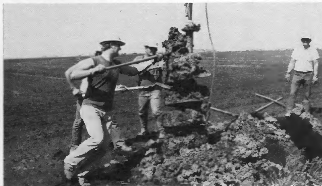
Muddy conditions caused considerable extra work for the construction crews.
