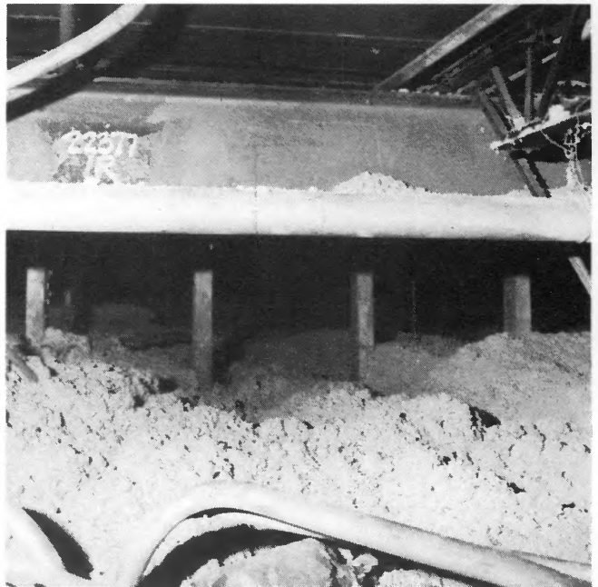
Eight inches of blown insulation has been added to the attic area.
