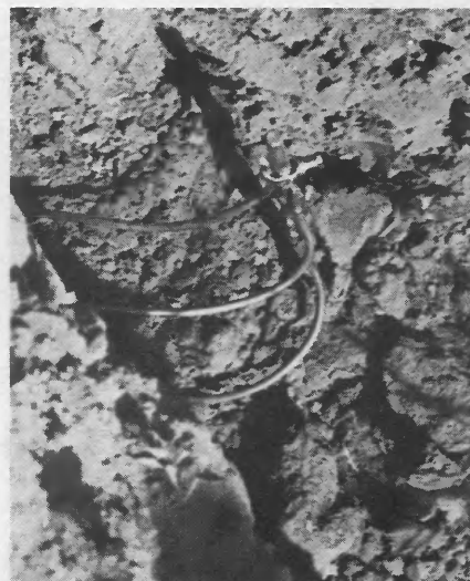
Grounding neutral on underground
