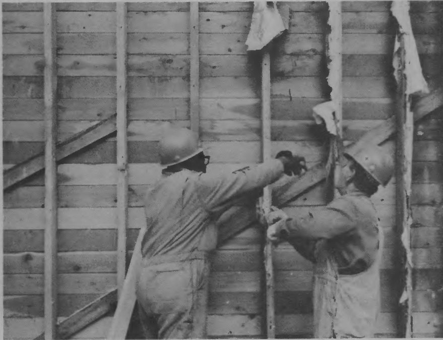
Far left: Jim Milligan, Raymond Smith and George Pyles put up paneling in the new community building at Carrier Mills. Center: Sandy Davis, District Director, and Fred Miller, Crew Foreman, inspect progress at a building being torn down for salvageable material to be used on weatherization projects in the Saline County area. Near left: Hobart Rollings and Charles Karnes begin disassembly of a building to salvage materials that will be used for weatherization projects.
