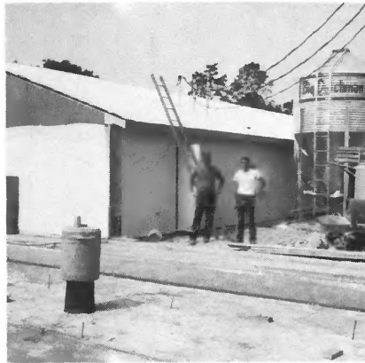
Showing building for gestation and breeding just finished, with one of the owners, John Meese, and Manager Darrel Mendenhall, left to right. (Oblong Pigs)
