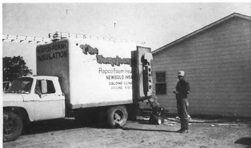
Rapco Foam insulation is being installed in new home by Newbold Insulation workmen.
