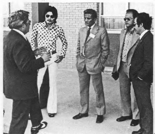
TOP: The trainees gave a cooperative line crew a hand with a sticky conduit coupling. ABOVE: Manager LeRoy Hard discusses the day with visitors, prior to an outing in St. Louis. RIGHT: The group watches a line crew finish wiring the transformer installation.
