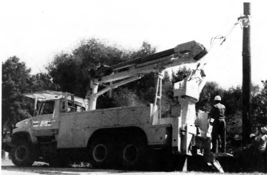
Clinton County Electric Cooperative employees help the city utilities of Carlyle and Breese with the setting of a 70-foot transmission pole.
