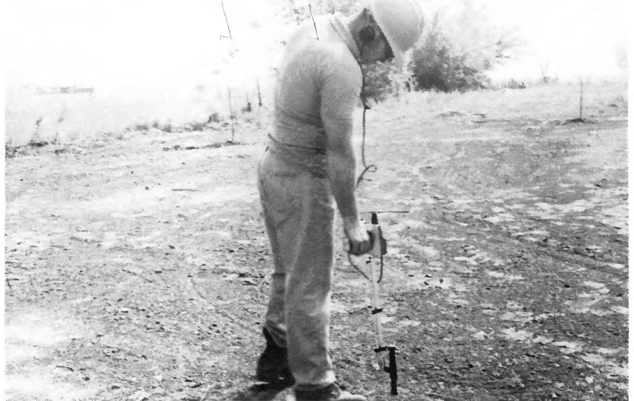
LOCATING WIRE—Lineman Albert Becker uses an underground line detector to locate buried cable prior to a contractor beginning to excavate.
