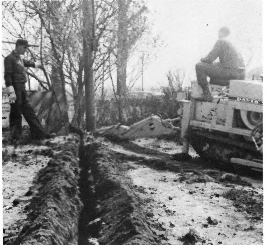
Employees Stan Timmermann (left) and Gene Edwards are with a trenching machine recently acquired by Clinton County Electric Cooperative for quick, efficient burying of some electric lines.
