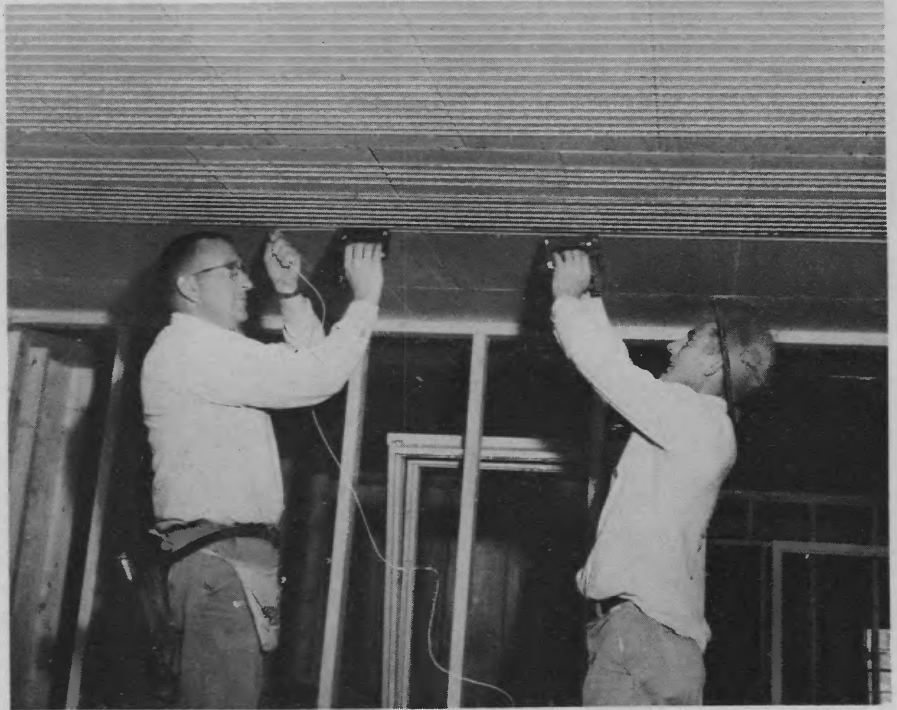
Mr. David Easterday, Nokomis building contractor, and his assistant, Alvin E. Bricker, install electric ceiling cable in another new home.
