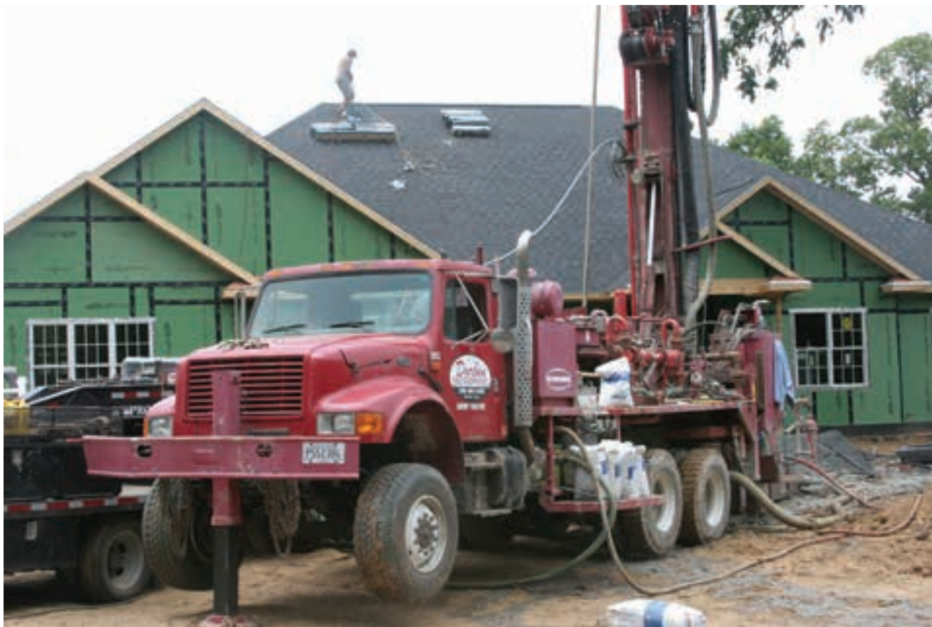
Holes are being drilled for a vertical loop installation which takes less land area.
