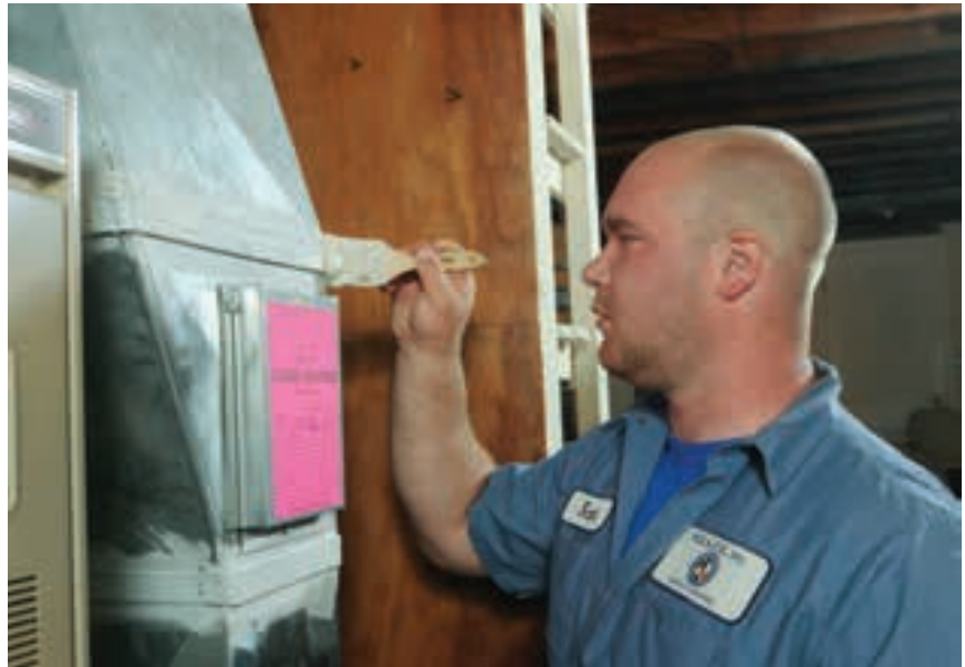
Mastic can be used to seal small gaps and leaks in your ductwork.
