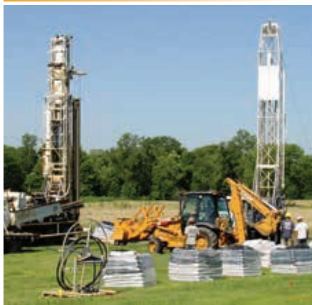
Installers work on a geothermal project at Southern Illinois University, one of 51 projects receiving funding under the GeoAlliance grant program.
