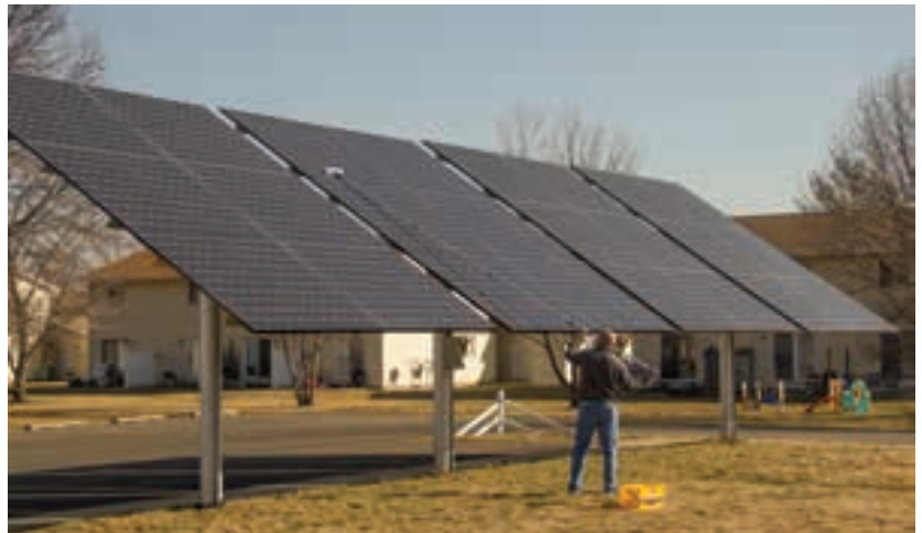
Electric co-op leaders agree with parts of the President's climate change plan announced in June, such as modernizing the electric grid and increasing the use of renewable energy from systems like this solar system owned by the Association of Illinois Electric Cooperatives. But they disagree with the carbon standard mandates that could raise rates an estimated 41 percent over the next eight years.
