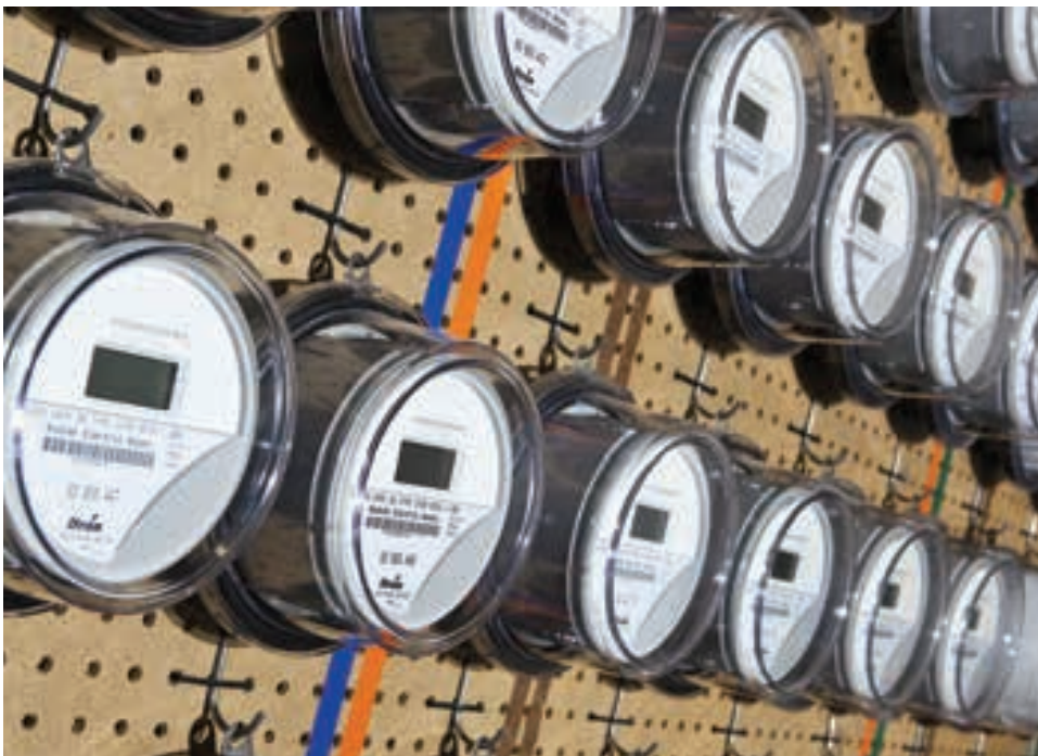
The proliferation of smart meters, along with other developing technologies, helps electric cooperatives work to contain costs while improving service for consumer-members. Source: NRECA
