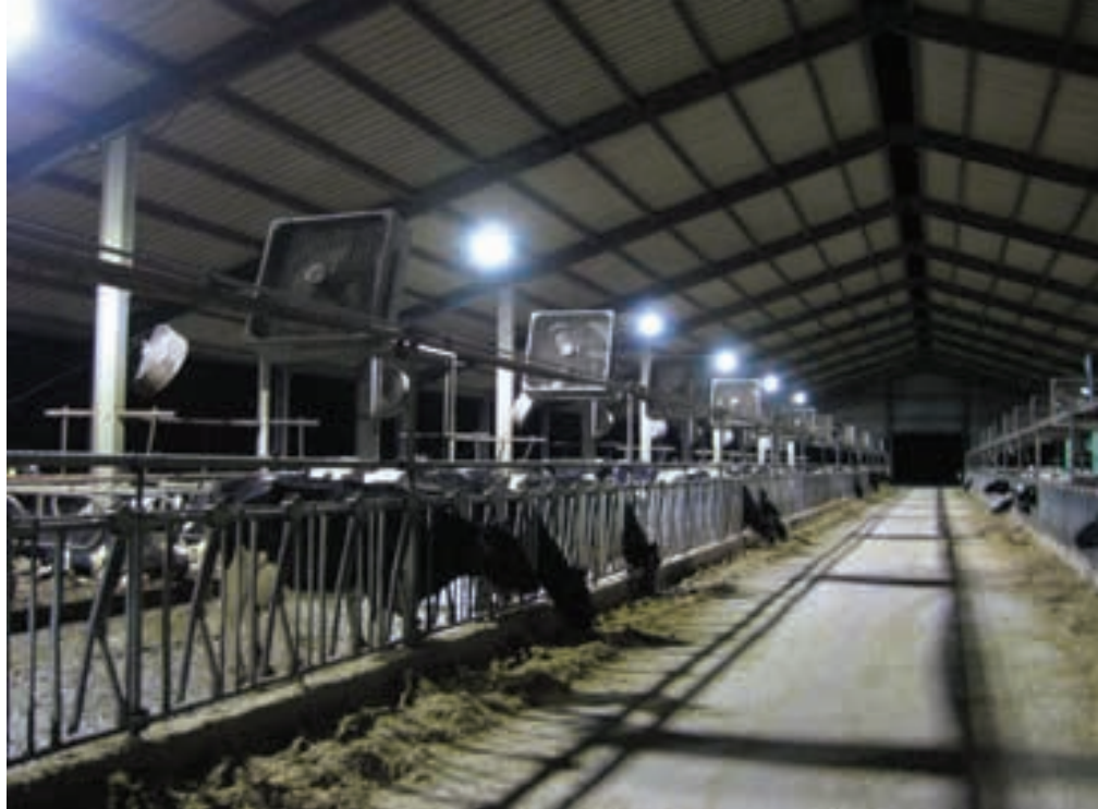
The T-Bar M Dairy Ranch, outside of Durant, Okla., normally uses 250-W metal halide lights in its barns. CRN exchanged those bulbs in 10 fixtures with 120-W LEDs. After six months, the dairy had cut energy use by 55 percent and boosted brightness by 30 percent. Source: Cooperative Research Network
