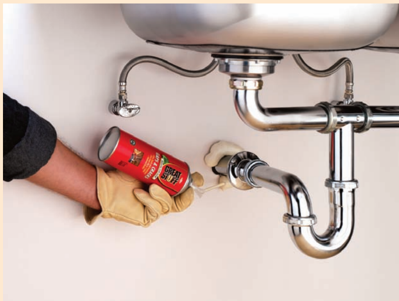
One of the most common areas that needs sealing is where plumbing pipes come through walls.
