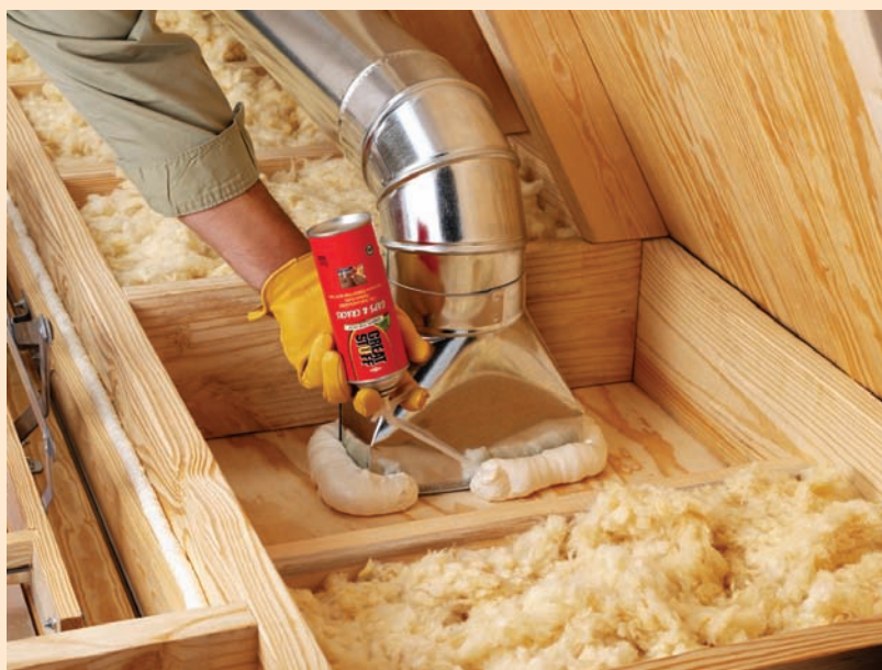
While sealing out drafts around doors and windows, look for hidden holes in areas such as your attic.
