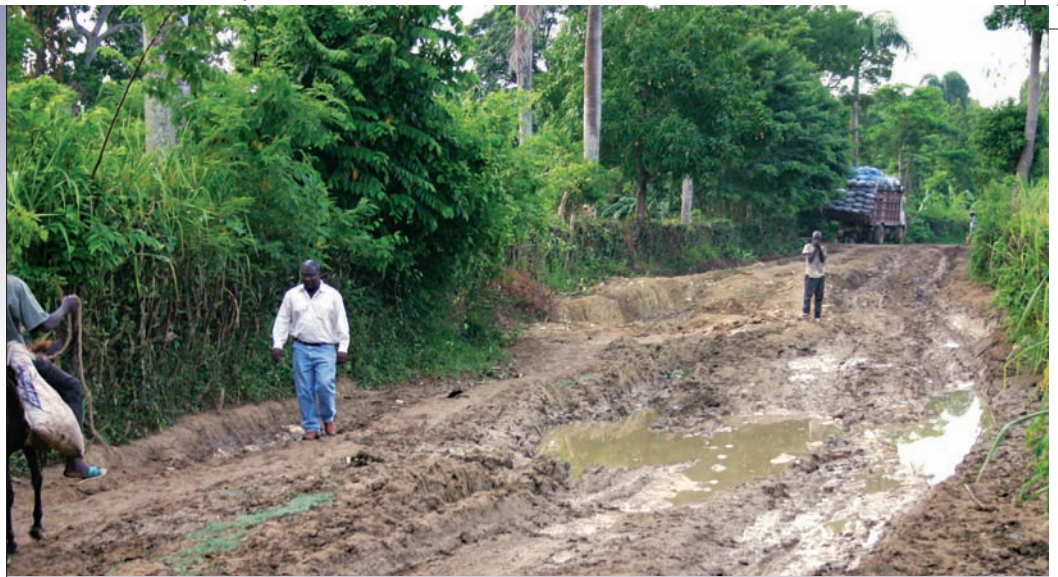
It takes hours to travel the "National Highway" in Haiti. Here it is seen a couple days after a rain. — Photo by Bruce Giffin
