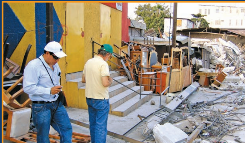
Myk Manon, head of the NRECA International emergency response team in Haiti, and Bud Stanley, inspect a downed power line on a street in Port-au-Prince. — Photo by NRECA International
