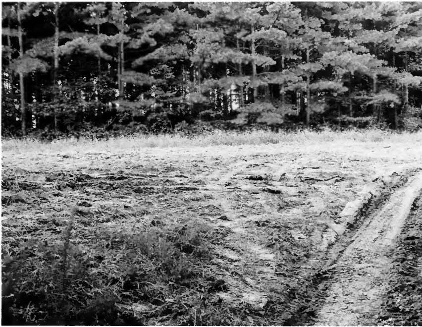
The right of way was damaged by four-wheel drive vehicles and had to be reseeded.
