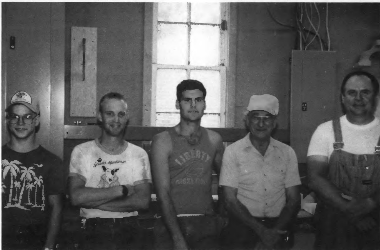
Workers at Concord Cabinets stand in front of the three-phase service panel that has helped make the expansion of the company possible. From left are Tony Huber, Brien Ohnemus, Steve Spilker, Wayne Sweeting and Gene Daggett.
