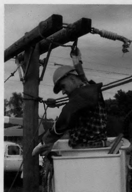
Preparing to take the line out of a suspension insulator, this worker will splice in a section of line.
