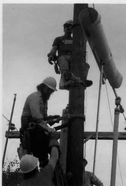
Much of the work is still done with muscle power. Here work is under way to lift up a pole arm.
