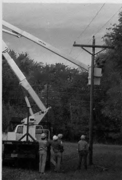
Under careful supervision, a Hot Line School student prepares to convert a three-phase line to single-phase.
