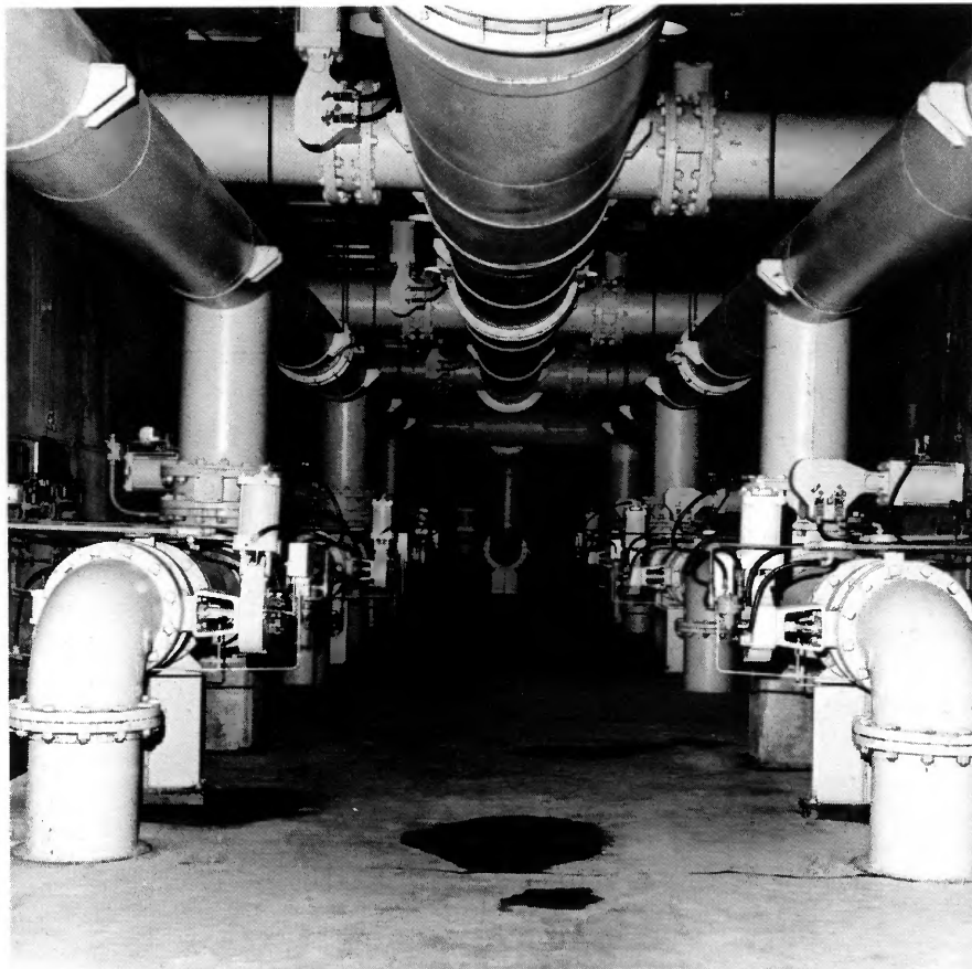
ABOVE: Huge pipes—called the filter pipe gallery—pumps water to and from filtering tanks at the Rend Lake water treatment plant. BELOW: A posterization of the Rend Lake Intra-City Water District plant. FAR RIGHT: Hopefully, water towers like this one will someday be sprouting up throughout Southern Illinois.
