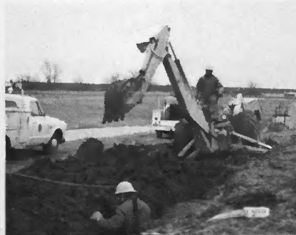
Underground distribution is installed at the Hidden Hills Subdivision by linemen of McDonough Power.
