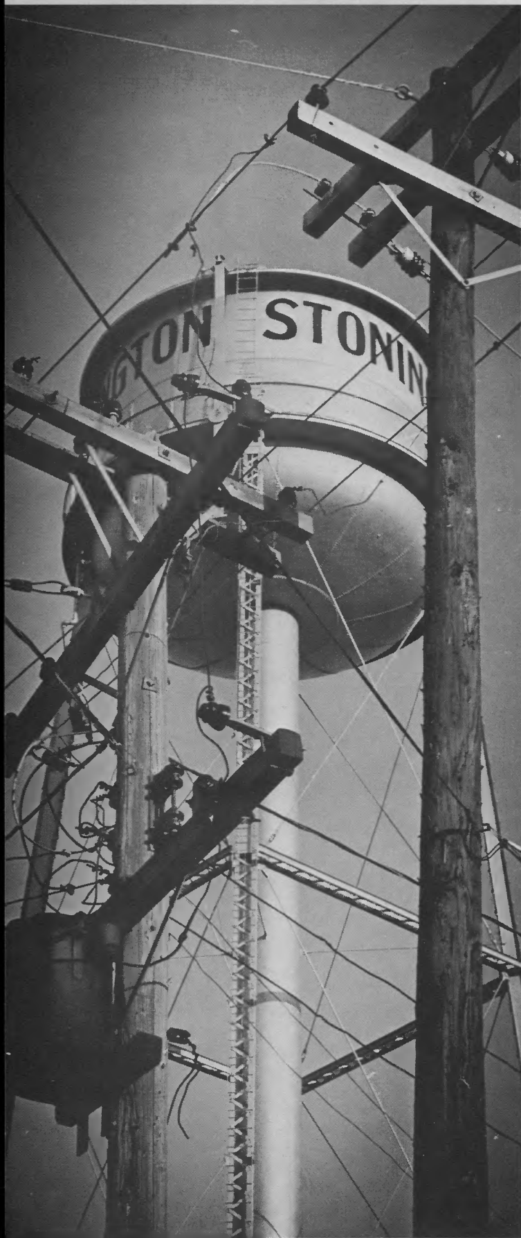
Old poles, old lines and old transformers throughout the thriving village of Stonington, near Taylorville, are to be replaced with a completely new distribution system—by Shelby Electric Cooperative, which henceforth will serve the town.
