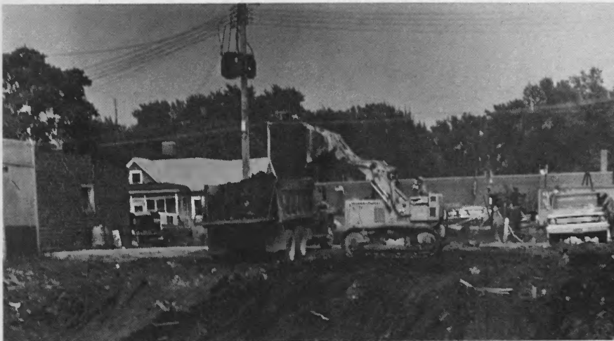
Excavation work on two former building sites prepared the site for Menard Electric's new headquarters addition.
