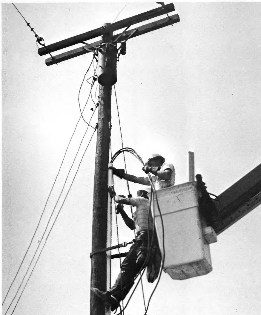
Skilled Wayne-White linemen run underground conductor from a transformer, down the pole to the already-prepared trench for another underground installation.
