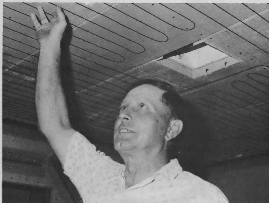
Raymond Heiser, Fisher, inspects electric heating system wires on the ceiling of his new home.
