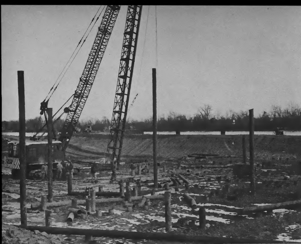
A crane is used to drive steel pilings 50 feet into the ground to support the substructure of WIPCO's generating plant under construction on the west banks of the Illinois River south of Pearl.
