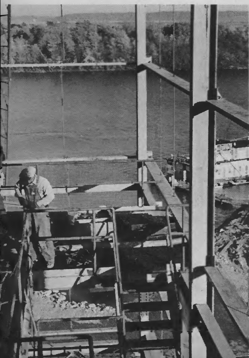
One hundred feet above the Illinois River workmen calmly take advantage of good weather to speed construction.
