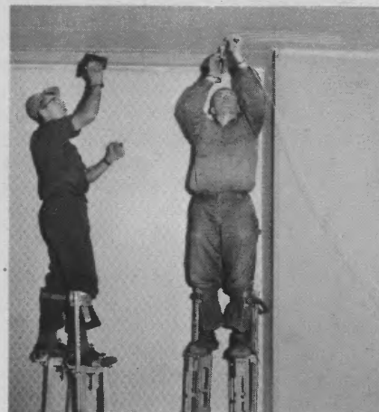
Electrician Wayne Rice (left) of Blue Mound and Kenneth Travis of Harristown, use stilts to staple electric heat cable on ceiling.
