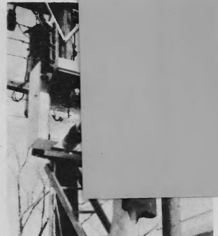
Inspector K. P. Branyan checking over the metering equipment at the Grade School in Cowden.
