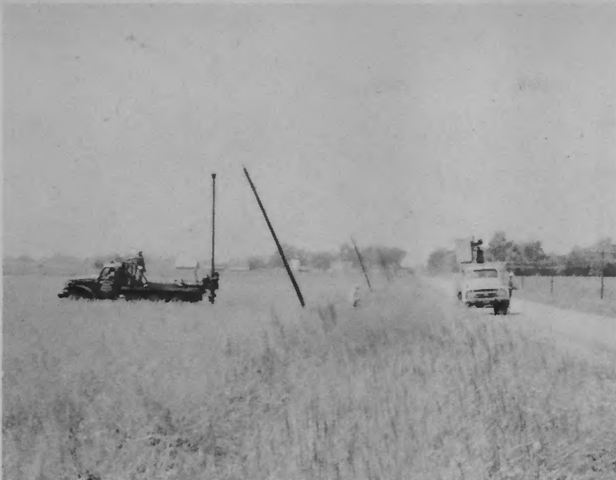
Cooperative crews leaning poles north of Cowden so that a new three-phase electric line can be built.
