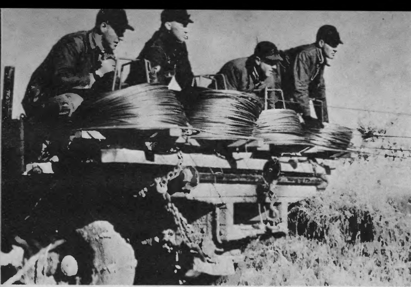
Crews stringing three-phase conductor—three hot and one ground wire—covered several miles in a day. Other crews put conductor on poles.
