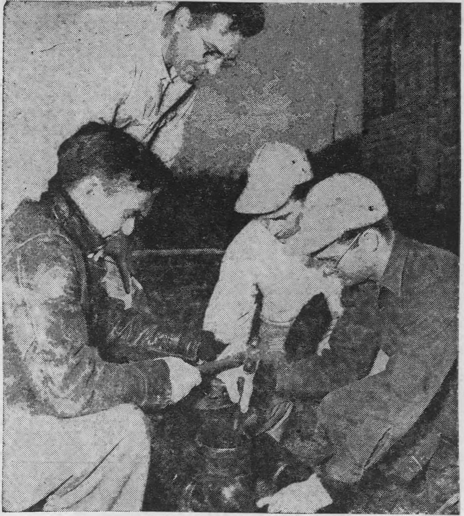
RECEIVING INSTRUCTIONS on how to fit drainage pipe together is this group of power use advisers, who attended the Illinois Power Use School, November 13-17, at Robinson. They are: left to right, Roy Goode of Rural Electric Convenience Cooperative of Divernon; Instructor Fred McVey of REA; Mel Wittenborne of Southern Illinois Electric Cooperative of Dongola; and James Sherwood of REA.
