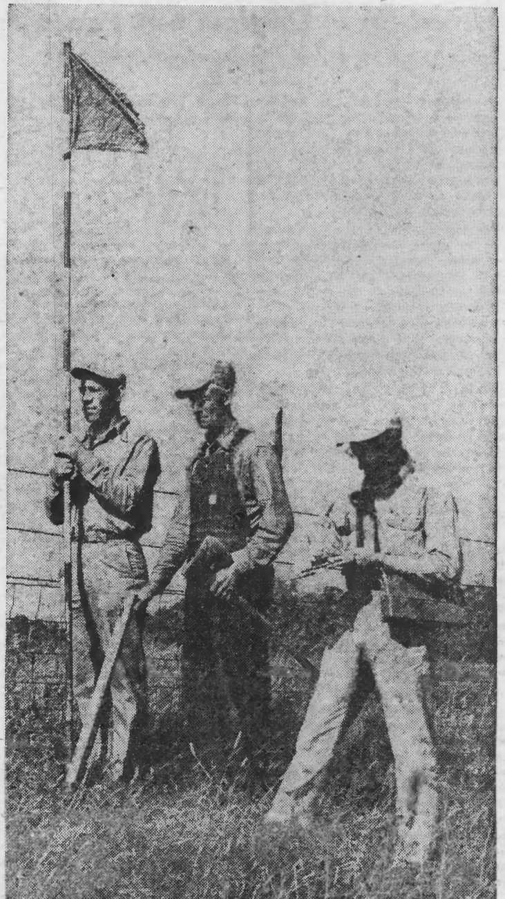
SURVEYING AND STAKING has been speeded up as much as 50 per cent. Instruction no longer have to be shouted. Rodman Dale Law, left, aligns rod with surveying instrument even though he can't see the instrument. Staker Iven Clark gets ready to hammer in stake, while Staking Crew Chief Harold Harkness keeps in constant contact over wireless phone with transit man.
