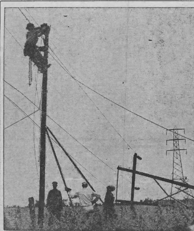
IN THE WAKE OF THE STORM—One of several wooden H-frames lies topped by the severe storm while linemen for the Mississippi Power company work to repair the damage. The 66,000 volt transmission line fell across Adams Electric cooperative's 3-phase feeder line one-third of a mile east of the co-op's sub-station on U. S. Route 24. The wires were suspended across the highway over the co-op's line. (Other pictures on Page 3)—Photo courtesy of Adams Electric Co-op.
