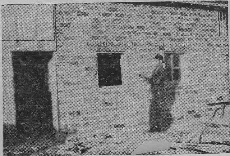
Shown above is the new slaughter house which is being constructed by the Golden, Ill., Locker cooperative on Route 102, about four miles southeast of Golden, and, going over his chart to see what equipment the linemen will need to complete an extension to bring electricity to the building, is Marion Young.
