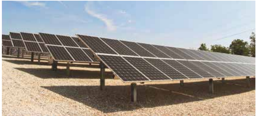
Prairie Power, Inc., a generation and transmission cooperative headquartered in Springfield, Illinois, plans to begin building solar farms in Illinois sometime later this summer. The project will include two 500 kW solar installations similar to this one built by one of its distribution cooperative owners, Illinois Rural Electric Cooperative in Winchester, Illinois.
