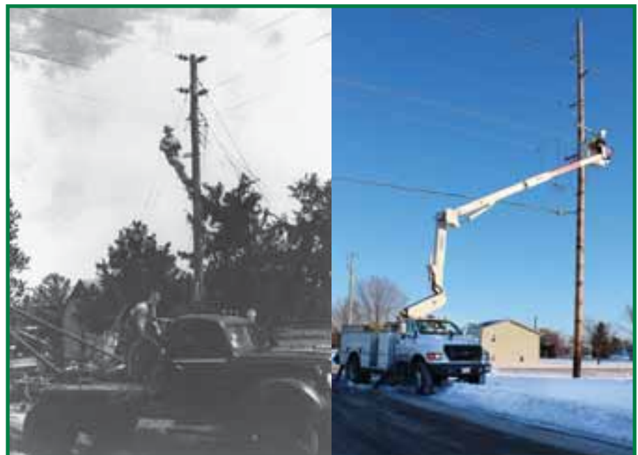
Back in the day line workers climbed a lot of poles and did most of their work while they were strapped to the pole. Today’s trucks have buckets attached to booms that lift workers up to the electric lines.
