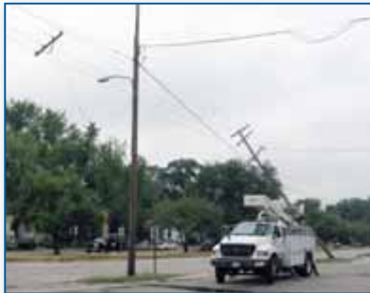
High winds during a July 24 storm caused extensive damage and a record number of outages. Poles on Blackhawk Boulevard in South Beloit were tipped, and some of the crossarms were disconnected.
