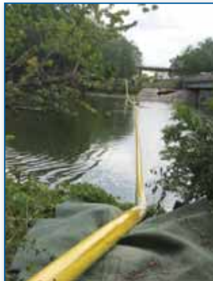
A natural gas pipe measuring about 700 feet was floated over the Rock River along Prairie Hill Road in South Beloit. After 40-foot sections of plastic pipe were melded together, workers used a stringing machine to pull the pipe across the river so it could be installed underground on the west side.
